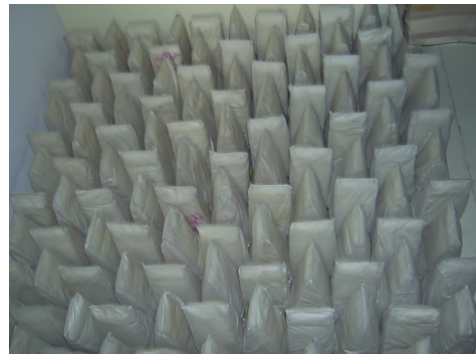
Glass wool wedges inside anechoic chamber
